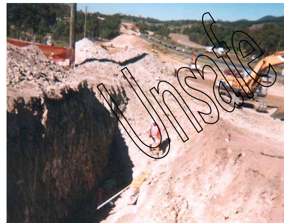
Unsafe trench – an example of what not to do
